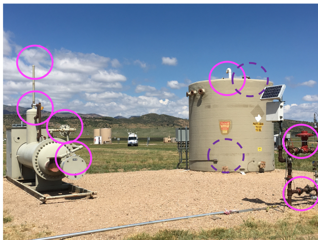
Figure 1. METEC facility with nine of the 11 release points circled. Release points include (clockwise from top of tank) tank candy cane, tank thief hatch, tank front flange, wellhead Kimray packing, wellhead hand valve packing, separator burner fuel supply, separator Kimray vent, separator pressure relief valve (PRV), and separator house PRV. Not pictured: wellhead lubricator flange and wellhead pressure gauge. The University of Wyoming (UW) mobile laboratory is in the background.
