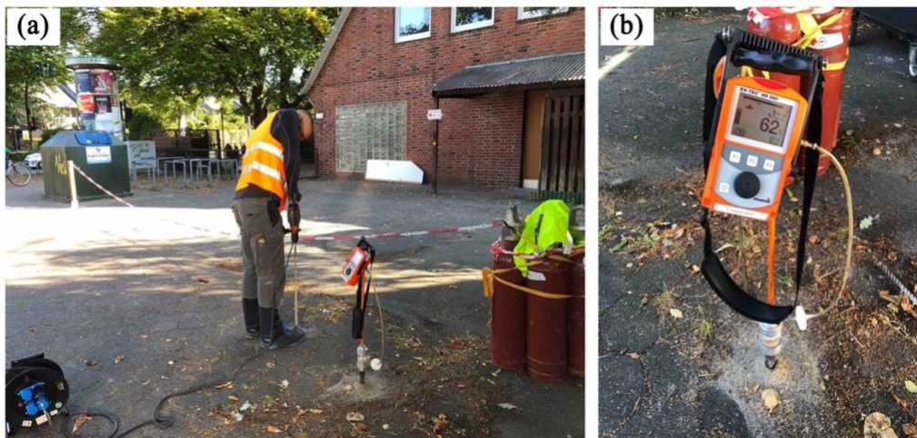
Figure S3 - Drilling holes around the surface-projected track of gas pipeline (a) and measuring the CH 4 mole percentage (b) to find the gas leak location, HH008
