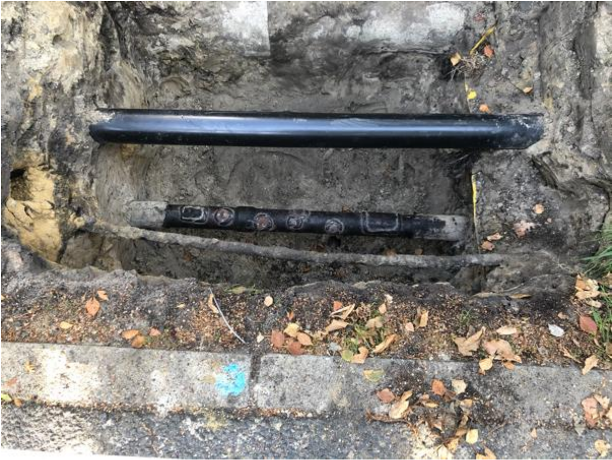
Figure S9 - The LDC reported 6 leaks on the pipeline at this location with total leak area of 5 cm 2 , HH013
