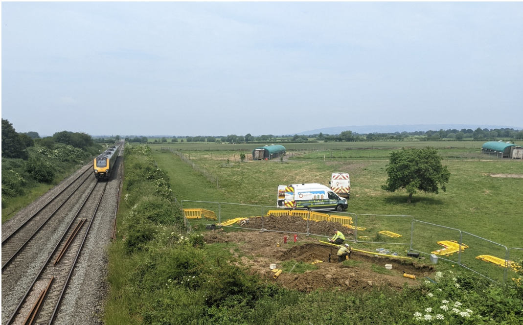
Figure S1. Image of gas leak site works taken on 12 th June 2023.
