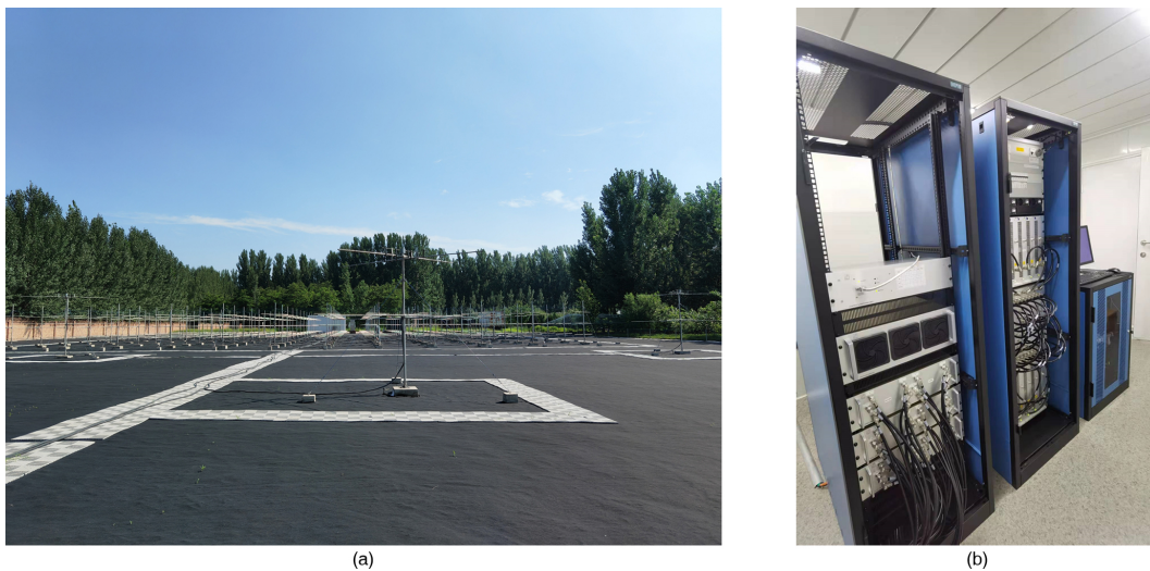
Figure 1. The photos of the new dual-frequency ST–meteor radar: (a) outdoor antennas and (b) DBS rack (left), Tx rack (middle) and Rx rack (right).
