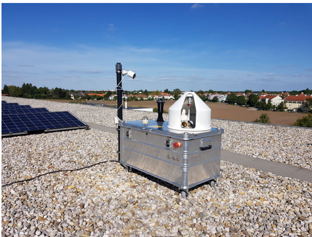
Figure 5. Image of the new enclosure system on the roof of a school at our southern site Taufkirchen. The systems includes, inter alia, the newly designed rotating cover, the lightweight aluminum case, the solar radiation sensor and a surveillance camera attached to a post.
