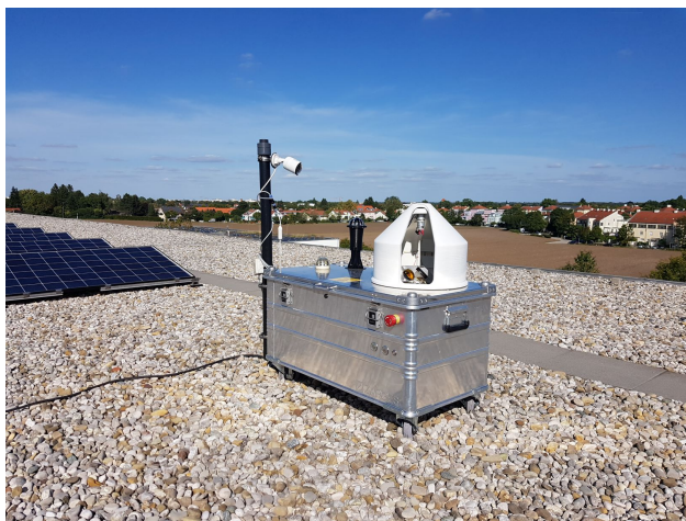
Figure 5. Image of the new enclosure system on the roof of a school at our southern site Taufkirchen. The systems includes, inter alia, the newly designed rotating cover, the lightweight aluminum case, the solar radiation sensor and a surveillance camera attached to a post.
