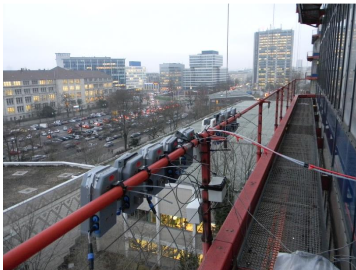
Figure 3. Set-up of the co-location of the prototype Zephyrs with reference instruments on the 6th floor of the Maths building. The grey units are the Zephyrs and the two inlet tubes connect to the reference devices located inside the office.
