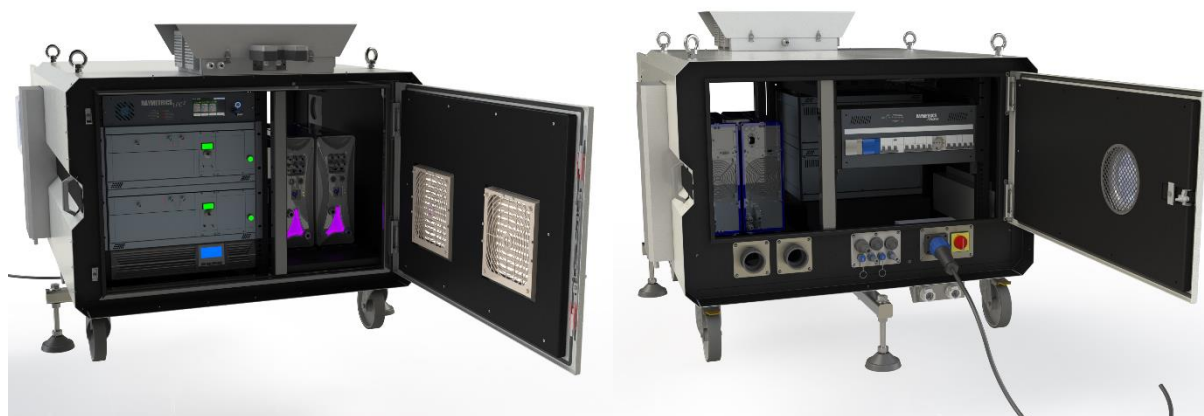
Figure 4: The front (left) and back (right) view of the electronics enclosure.
