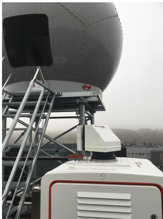
Figure 1. Vaisala WRS400 X-band radar and WindCube400S Doppler lidar installed on the roof of a building at Vaisala Oyj headquarters in Vantaa, Finland. Photo taken by Raisa Lehtinen.
