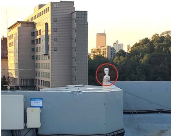
(a) Surveillance camera
