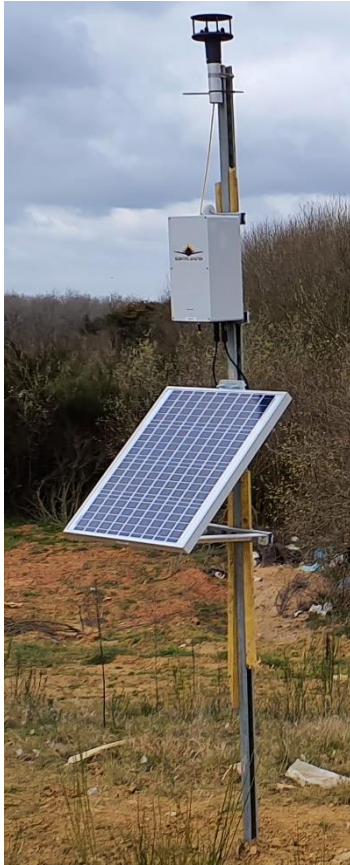
Figure 3: System A autonomous field logger (LSCE007) installed at the SUEZ Amailloux landfill site in March 2021 (see text for description). This system includes a two-dimensional anemometer.
