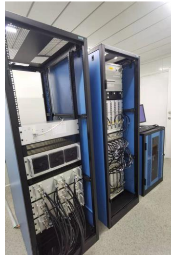
(b) DBS rack (left), Tx rack (middle) and Rx rack (right)
