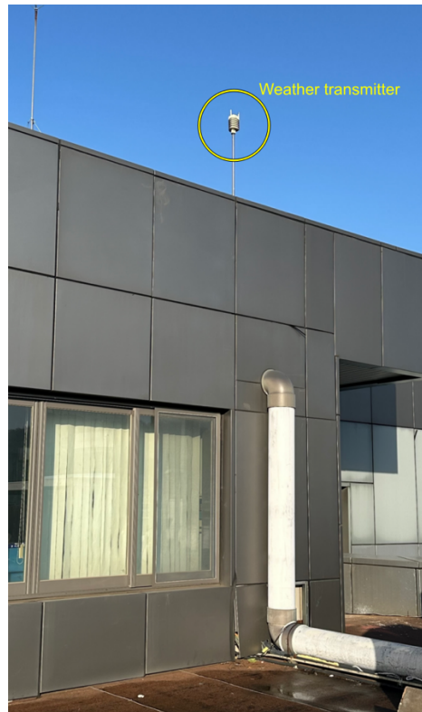
Figure 3. Installation of the weather sensor (WXT510) on the roof of the building
