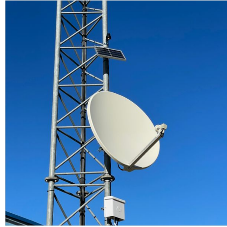
Figure 2. Image of a sensor installed by HD Rain on a mast of a fire brigade building (commercial collaboration with the SDIS, departmental fire and rescue service) with in the south of France
